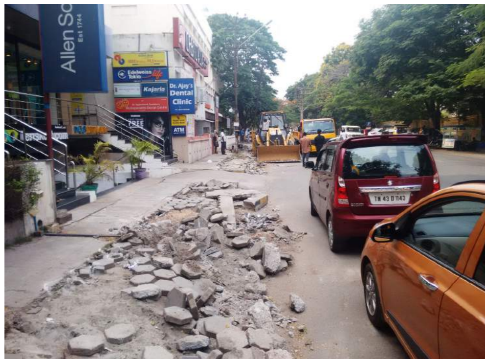
Fig. (above) Debris being cleared from DB Road in Coimbatore
