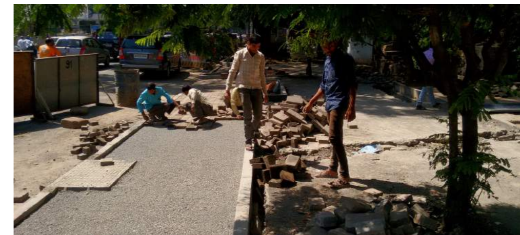
Fig. Paving tiles/blocks are laid on the compacted base to finish the footpath. This requires fine workmanship to ensure that the blocks are laid close together and do not come loose in the future.
