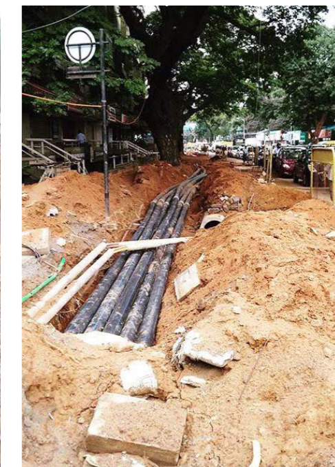
Fig. (left) Damage caused by excavating beyond 2 m around trees in Coimbatore
