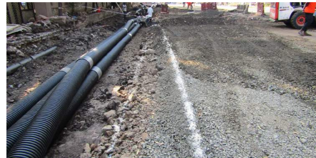
Fig. (top left) Workers manually levelling the granular sub-base in DP Road, Pune
