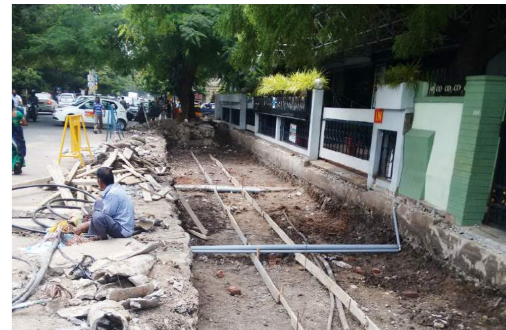
Fig. (above) Excavation work carried out in Coimbatore ahead of the rainy season to prevent stagnation of water
