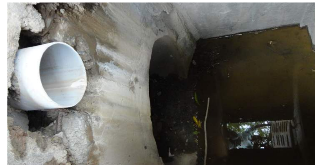
Fig. Manhole with catchment pit opening in DP Road, Pune
