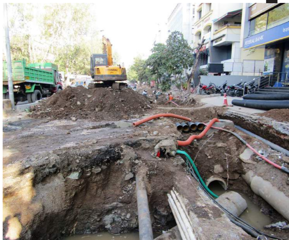
Fig. Complex network of existing underground utilities at different levels in DP Road, Pune
