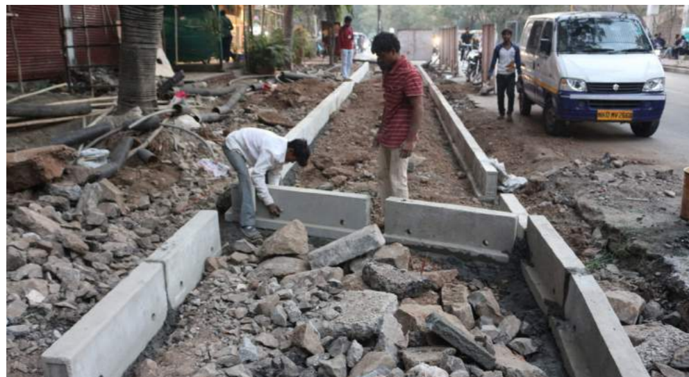
Fig. (above) Alignment of kerb stones as per design in JM Road, Pune
