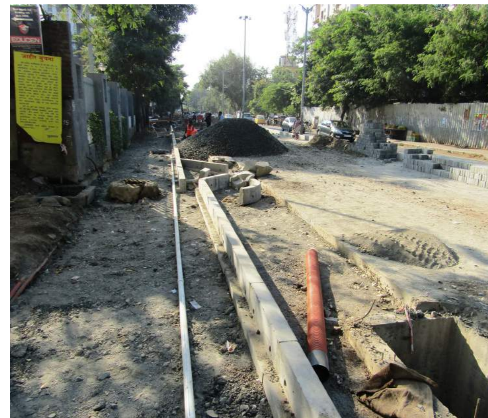
Fig. (above) Kerb stones are carefully placed over PCC mortar base maintaining the alignment and height in FC Road, Pune
