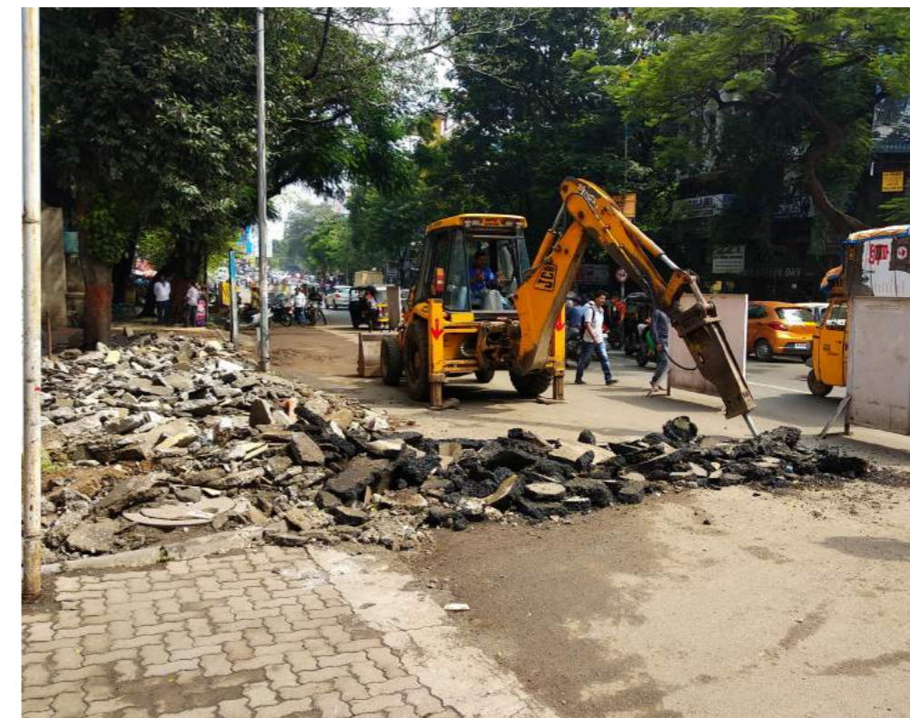
Fig. (above) The site is marked to be demolished/scarified/ excavated at ITI Road in Pune
