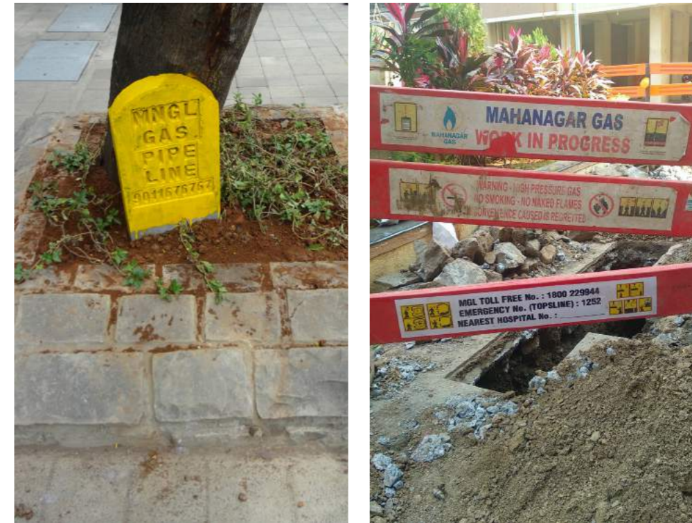
Fig. (left) Gas mains and utilities carrying combustible material
